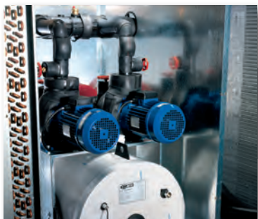
dual pumps & storage tank
